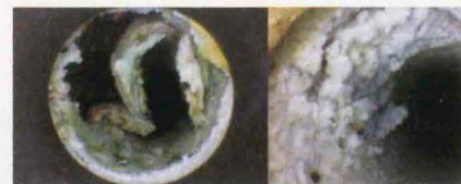
Fig. 2: Internal borescope images revealing the decomposition of the interior plastic tubing.
