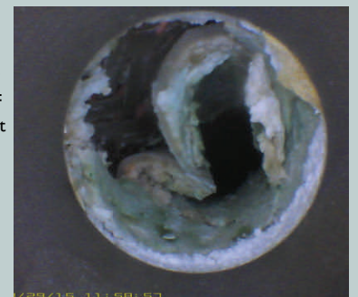
Internal borescope image revealing the decomposition of the interior plastic tubing.
